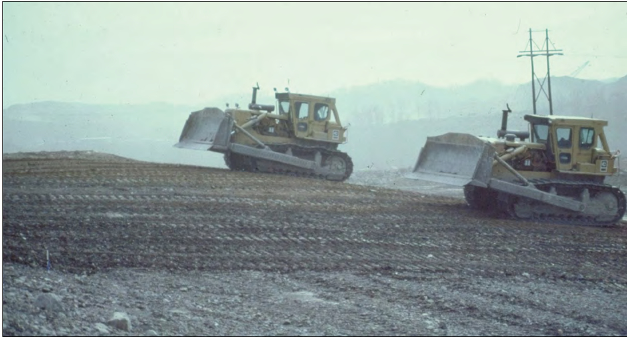
Figure 2-4.—Soil compaction due to heavy equipment operation on mine soils hinders survival and growth of planted trees. “Tracking-in” operations, such as those shown in the photo, are not recommended for mine sites on which trees will be planted, unless required to stabilize steep slopes. Photo by J. Burger, Virginia Tech, used with permission.
