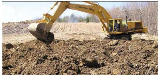
Figure 3-9.—Excavator leveling dumped topsoil piles. An excavator can be used to level soil piles without causing compaction and can be useful when the dumped soil piles contain stumps, logs, and other coarse woody debris. Photo by J. Burger, Virginia Tech, used with permission.
