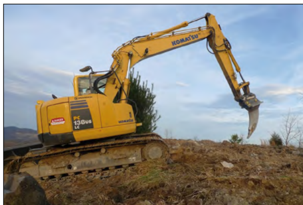
Figure 10-5.—An excavator outfitted with a ripping tooth. This equipment can loosen compacted soils on slopes that are too steep for a dozer. Photo by N. Hall, Green Forests Work, used with permission.
