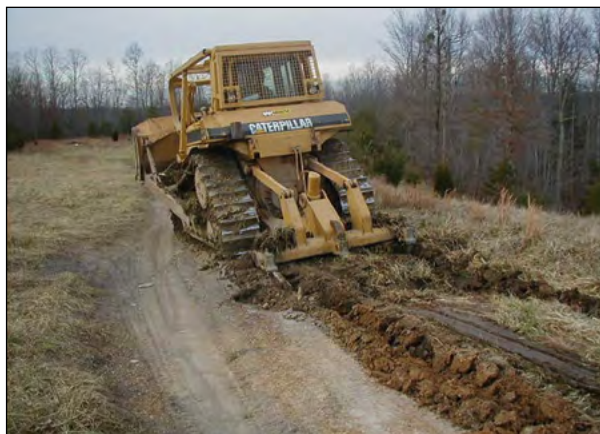
Figure 5-2.—A dozer ripping to loosen soils and produce soil conditions favorable to successful reforestation in a former roadway. Photo by P. Angel, OSMRE.
