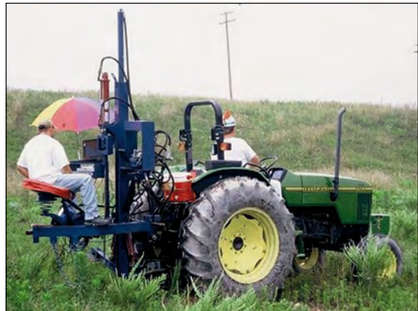
Figure 5-7.—A tractor-mounted cone penetrometer being used to evaluate soil density on a Kentucky surface mine. Photo by OSMRE.
